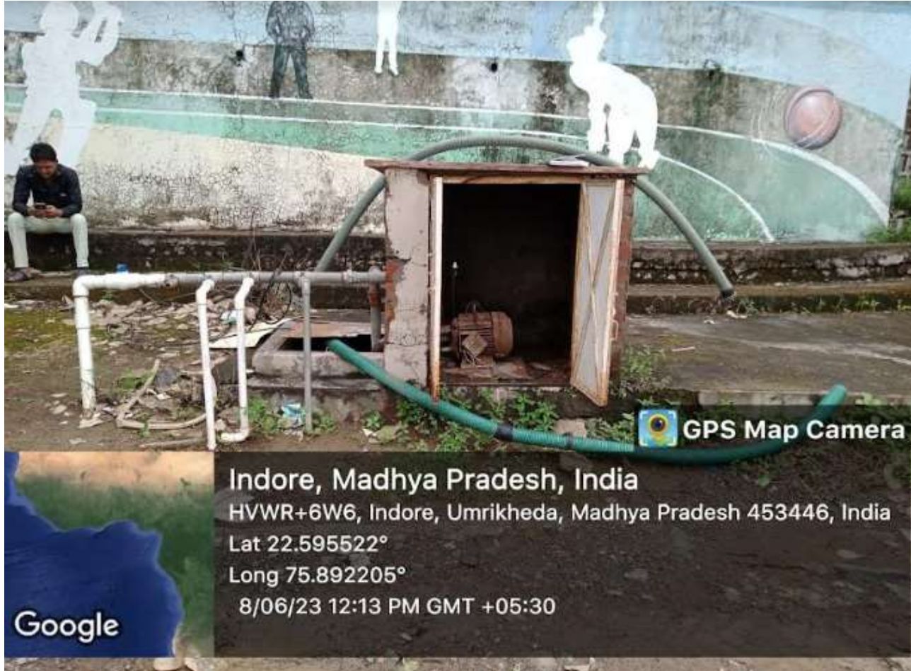
Fig. 2.2 Fresh water pumping station
