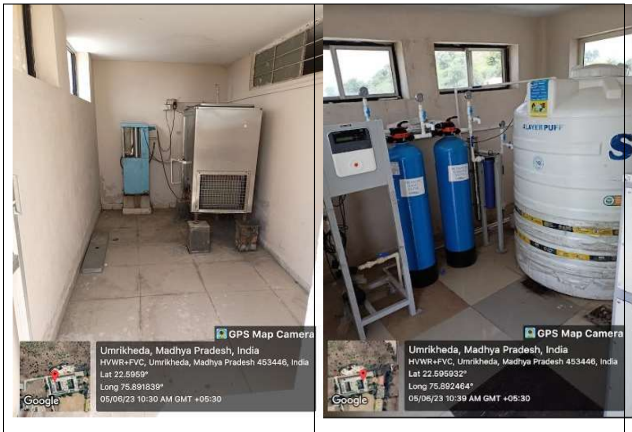
Fig: - 2.6 Water Filters for drinking water in Institute campus
